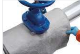
Figure 57: Wrap around flanges to enclose valve and wire in place.
