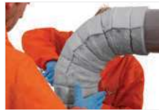
Figure 37: Push all gores together to ensure there are no gaps at joints and tighten wires.
