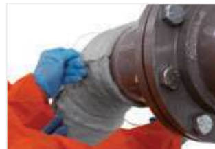
Figure 35: Ensure all joints are closely butted without gaps and that they fit the pipe tightly without voids.
