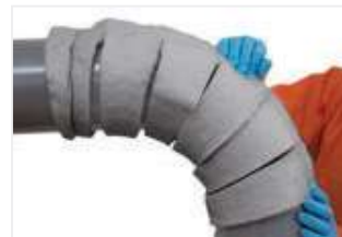
Figure 39: Position cut outs on inside throat of bend with longitudinal joint on outside of bend.
