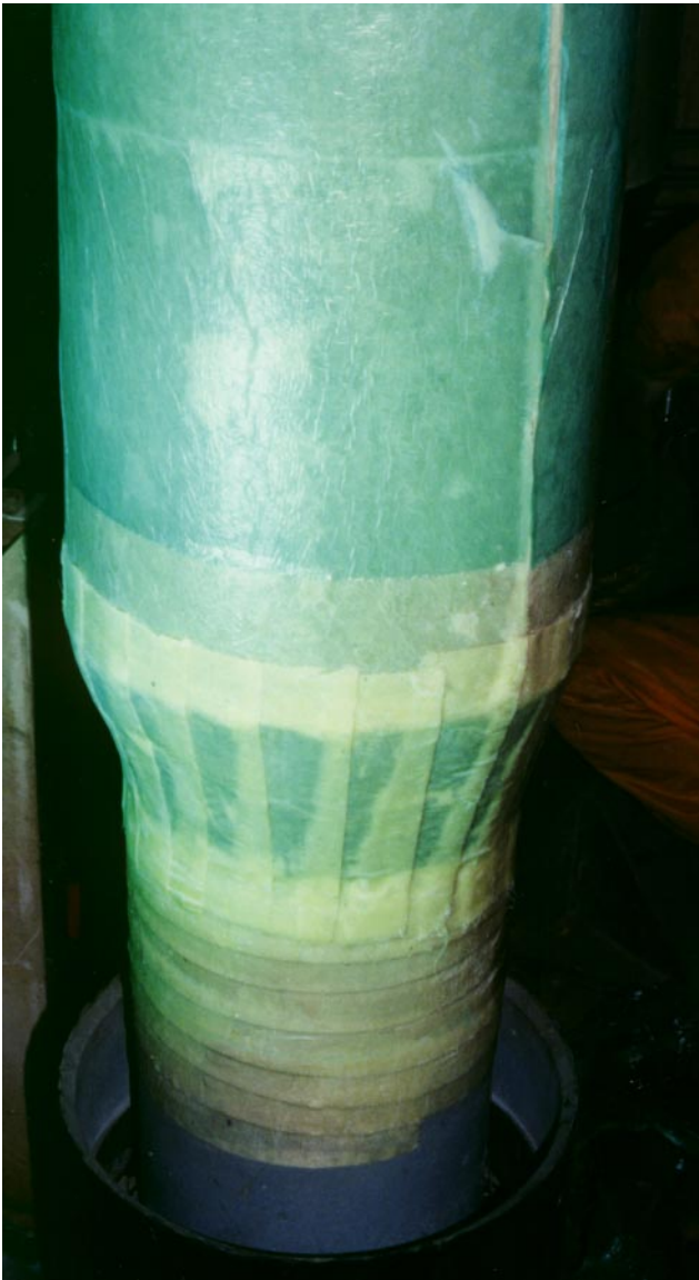
Pic. 12 Insulated Riser wrapped in Fibaroll - showing termination to coated pipe - curing in progress
