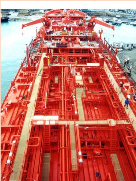
Protection insulation on pipework (overpainted) on chemical tanker - Italy
